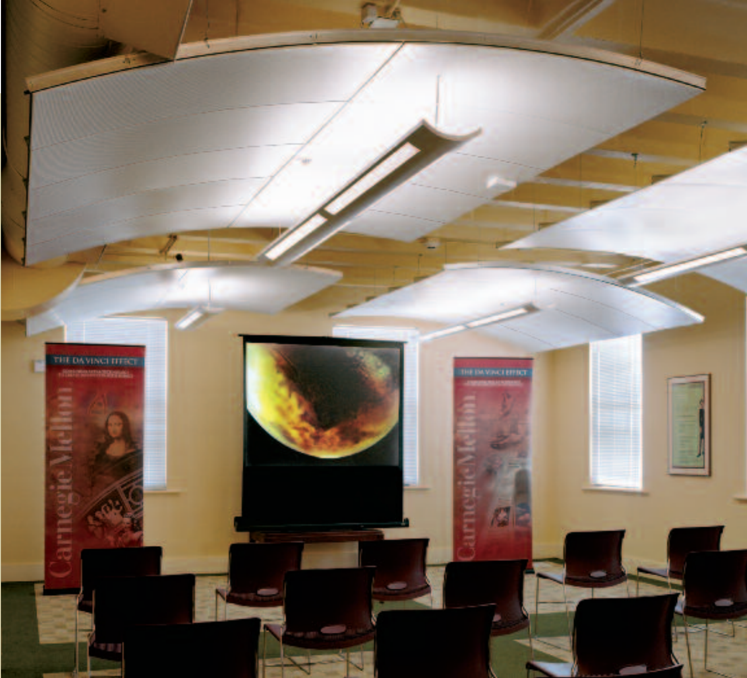
Above: Carnegie Mellon at NASA Ames Research Center, Mountain View, CA Architect: Architectural Resources Group Product: Curved Solutions 250, color: Cotton White
